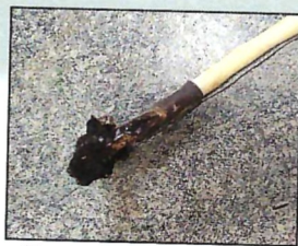
Burnt Out Cable
